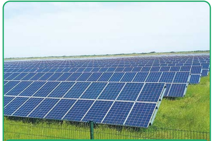
1.1 MW JHALERA, HIMACHAL PRADESH
