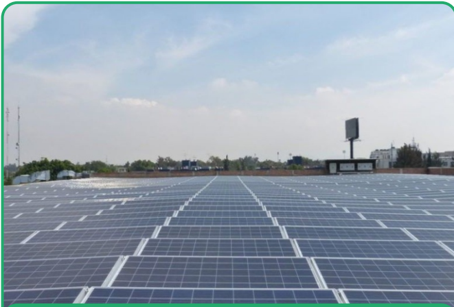
1.75 MW X 2 VIJAPUR, GUJARAT
