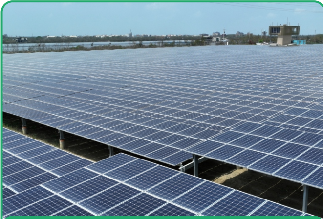
6 MW AT GUJARAT
